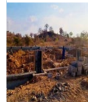
EXTERIOR STUB COLUMNS FINAL SHATTERING
